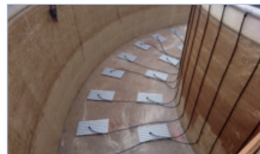
Aeration elements of an aeration basin
