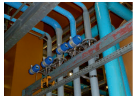
Vortex flowmeters measuring compressed air
