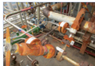
Retrofitted flange pressure tapping
