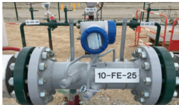
OPTISONIC 7300 ultrasonic flowmeter prior to commissioning
