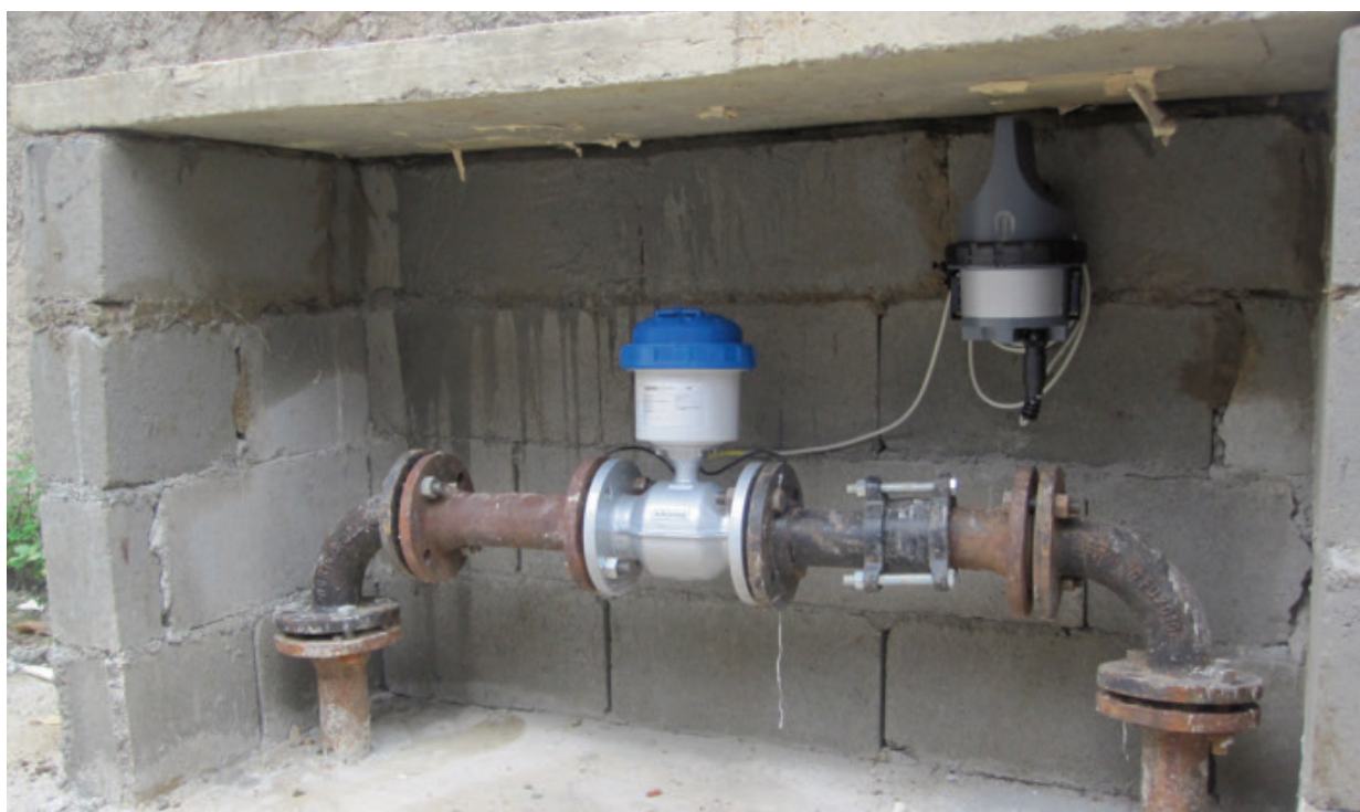
WATERFLUX with GPRS module KGA 42 in aboveground part of the pipeline
