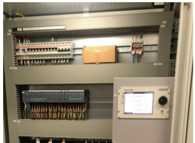
SUMMIT 8800 flow computer in control cabinet
