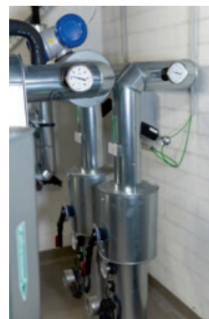
WATERFLUX 3300 measures the return flow to the geothermal probes
