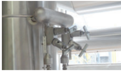
Venturi nozzle installation
