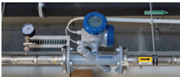
Flow measurement of natural gas for the humidifier
