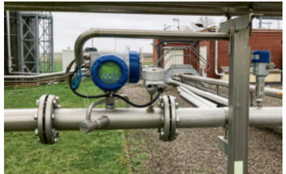
OPTISONIC 7300 Biogas ultrasonic flowmeter and OPTIBAR PM 5060 pressure transmitter installed at the outlet of the digestion tower
