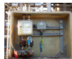
Previous DP transmitter before replacement
