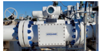
Custody transfer flow measurement of natural gas
