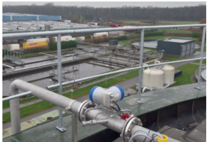
Flow measurement of biogas behind the digester
