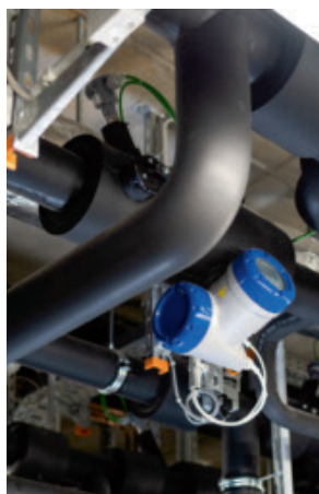
Electromagnetic flow measurement of hot water
