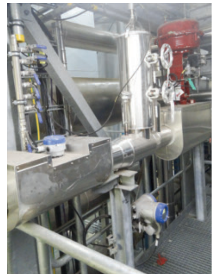
Feedwater measurement with the OPTISONIC 3400 ultrasonic flowmeter
