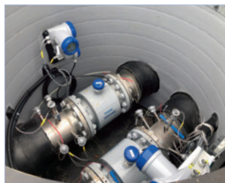
District heating measurement with OPTISONIC 3400 District Heating flowmeter, OPTITEMP TRA-T30 temperature sensor and OPTIBAR PM 3050 pressure transmitter
