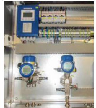
Control cabinet with KROHNE DP and pressure transmitters, temperature transmitter and flow computer
