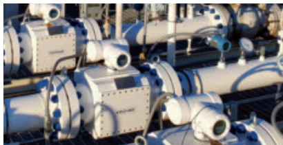
Gas fuel skids with ALTOSONIC V12 ultrasonic gas flowmeters
