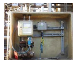
Previous DP transmitter before replacement
