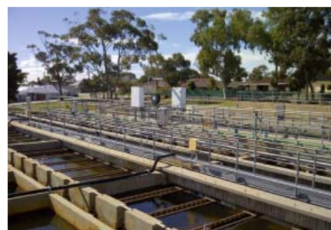
Sludge level monitor installed on sedimentation tank
