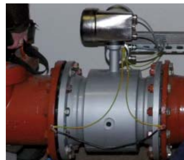
TIDALFLUX 2300 F in the discharge to the mixed water drainage system
