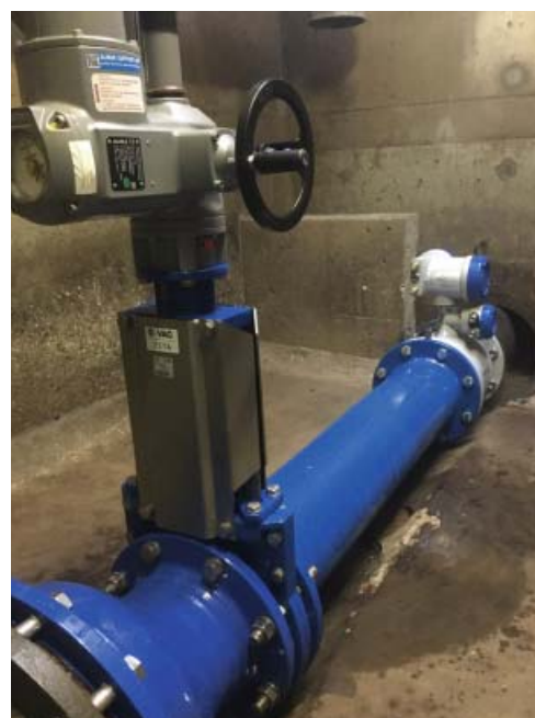
Measuring solution including flowmeter and slide valve
