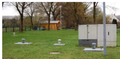
Transfer of measuring signal to the control cabinets
