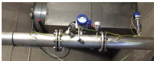
The OPTISONIC 7300 Biogas installed behind the filter
