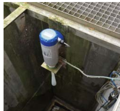
OPTIWAVE 5200 C above the wastewater container
