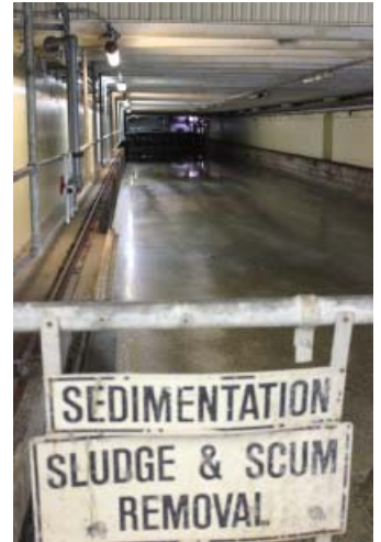
Primary sedimentation tank
