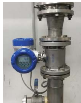
Flow measurement of fat for pump control
