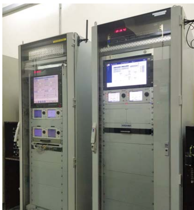
Supervisory control cabinets equipped with SUMMIT 8800 flow computers and SynEnergy software
