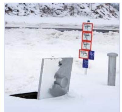
Entrance to a distribution shaft
