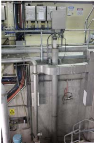
OPTISYS SLM 2100 mounted on a hopper of a primary sedimentation tank
