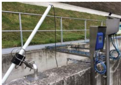
Turbidity measurement in the effluent channel
