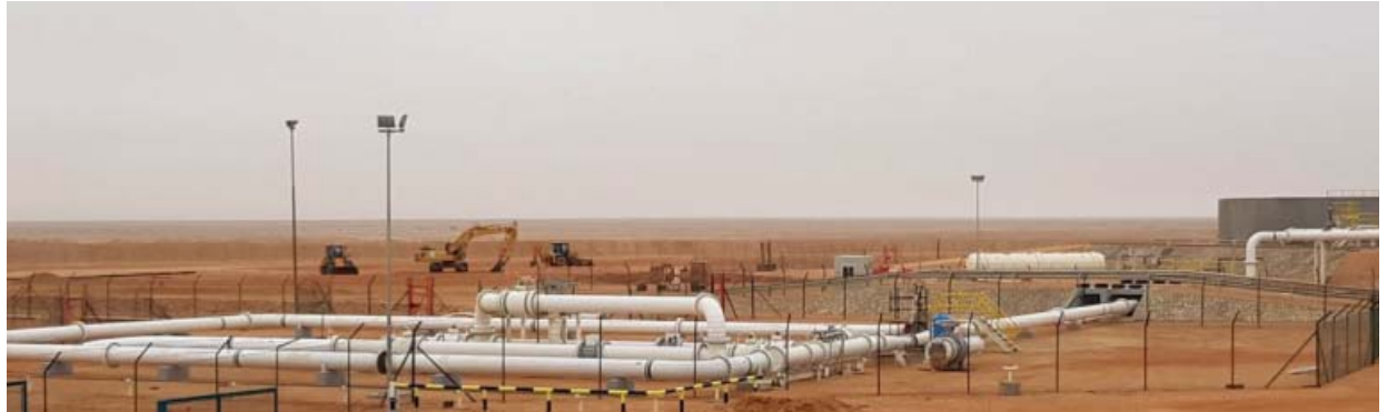
Treatment plant with water skids
