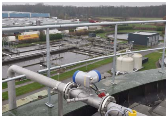
Flow measurement of biogas behind the digester
