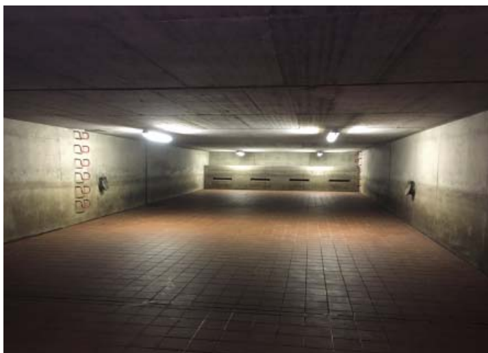
Underground storm overflow basin in the Municipality of Schlangen
