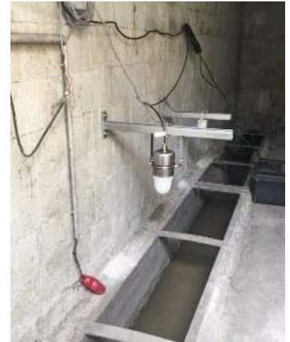
OPTIWAVE 1400 suspended above the open channel
