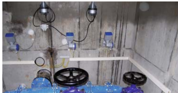
3 WATERFLUX 070 F converters and 2 KGA 42
