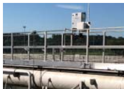
Measurement of sludge level
