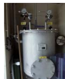
Gas inlet with first water separator
