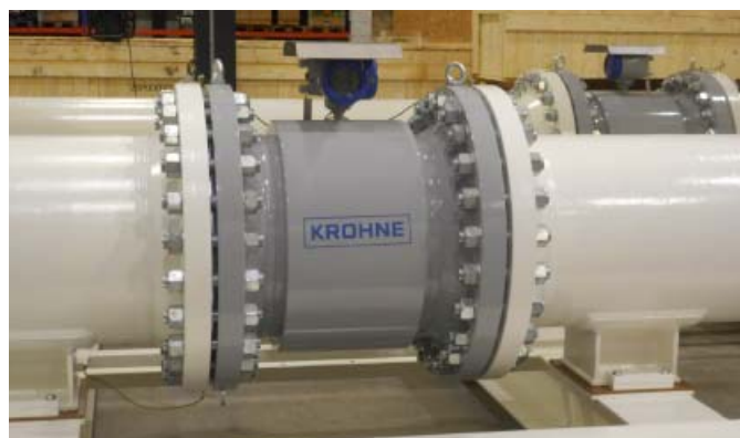
OPTIFLUX 2300 installed on water skid
