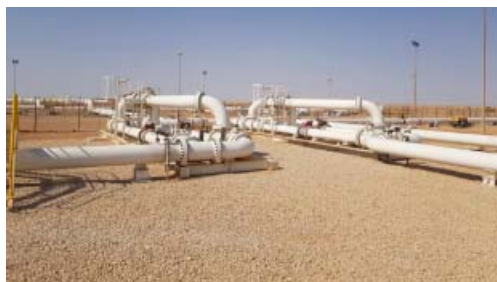
Both water skids installed side by side
