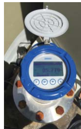
OPTIWAVE 6500 C installed on top of the lime silo
