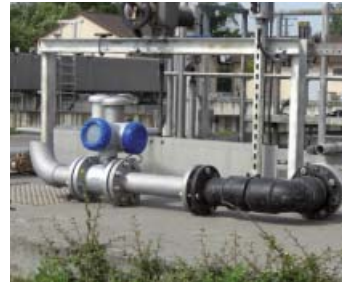
Test set-up at a sewage treatment plant
