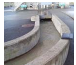
Open channel from grit chamber to preliminary clarification
