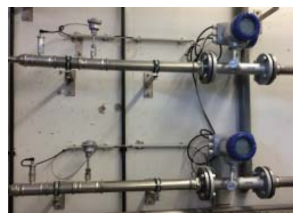
Compressed air measurement
