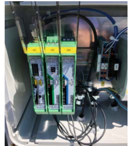
Wireless and I/O modules for the KRL 70 transmitting unit on the scraper
