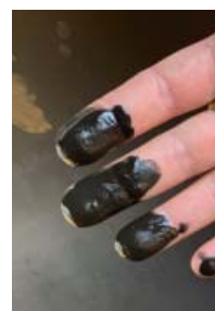
Media leaking from inside the coil housing
