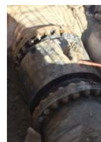
Damaged EMF before replacement
