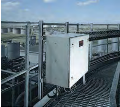
Installed LAND FGA
