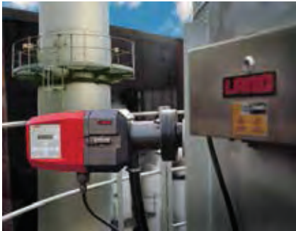
Installed Model 4500 MkII+
