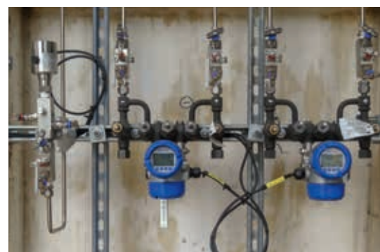
Pressure transmitter at a biomass plant
