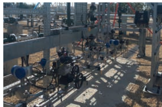
Hydrogen mass flow measurement
