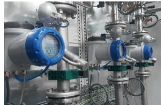
Flow measurement of natural gas and oxygen for combustion control
