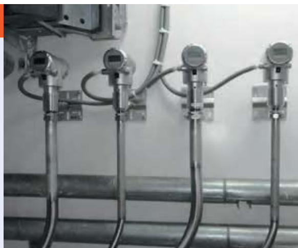
TDR level measurement of condensates in irradiating environment
