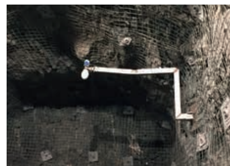
Level monitoring in an ore pass
