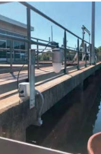
Radars level measurement of water basin
