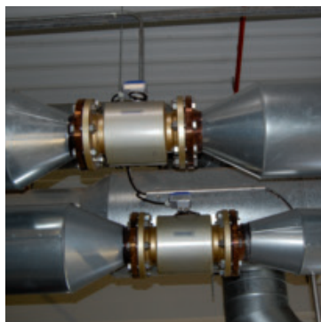
Measurement of the hot water in the brewing house
