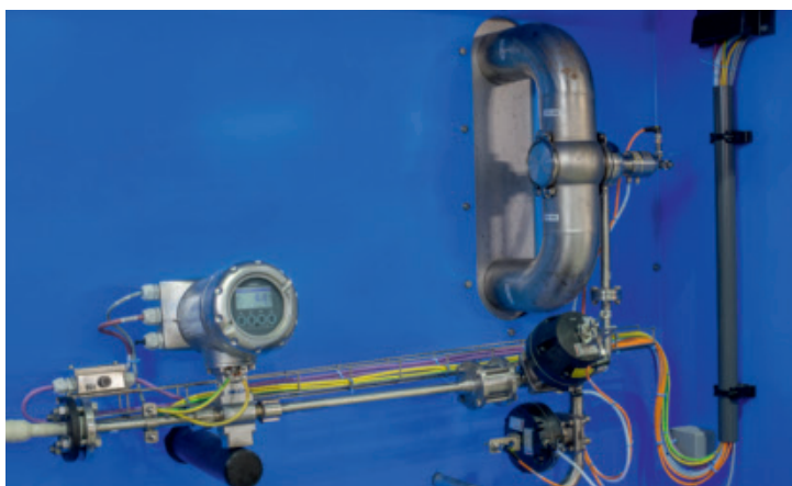
Process instrumentation for the CIP (Clean in Place) system: Stock management with the OPTIFLEX 2200 level transmitter (top and centre left). Dosing of CIP agents (bottom) and flow measurement of the CIP lines (top/centre right).
