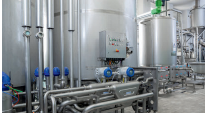
Installation of the OPTIMASS 6400 in front of the buffer tank
