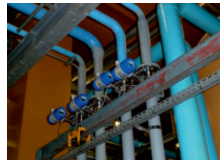
Vortex flowmeters measuring compressed air
