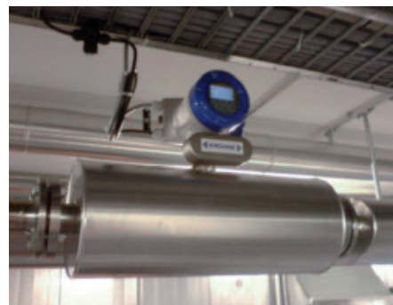
OPTIMASS 1300 C in a vegetable oil pipeline
