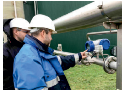
Measuring device start-up carried out by a KROHNE service technician
