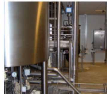
CO 2 recovery plant
