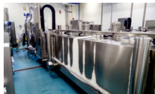
Tunnel freezer for cryogenic freezing of goat cheese
