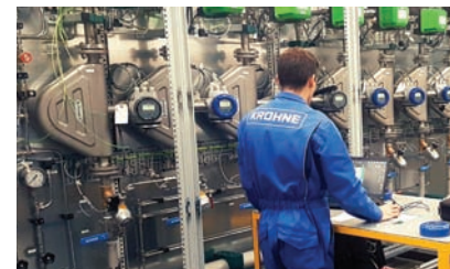
Combustion control cabinet with OPTIMASS 6400 Coriolis mass flowmeters for oxygen measurement
