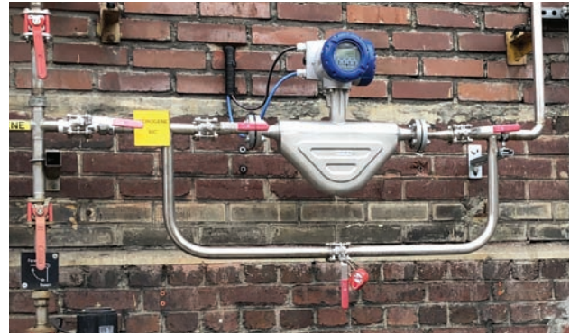
Hydrogen measurement at MERSEN with the OPTIMASS 6400 Coriolis mass flowmeter (DN10)
