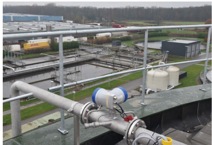
Flow measurement of biogas behind the digester
