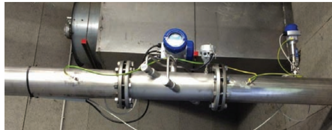
The OPTISONIC 7300 Biogas installed behind the filter
