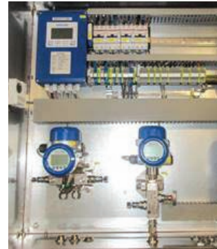
Control cabinet with KROHNE DP and pressure transmitters, temperature transmitter and flow computer
