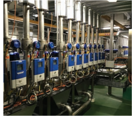
Flow measurement of beer with OPTIFLUX 6300 W (installed near beer tank)
